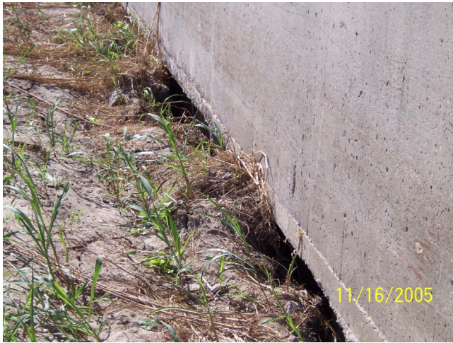
Fig. 1. Photograph of gap on canal side of Michoud Canal I-wall in New Orleans after Hurricane Katrina
