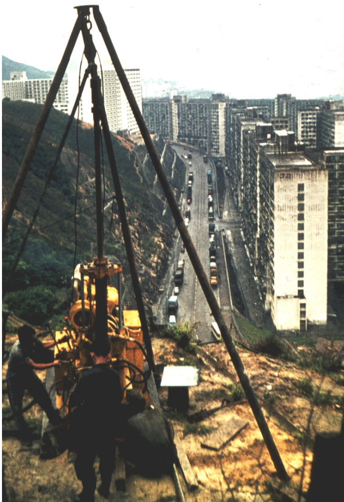
Figure 11: Drilling vertical diamond core holes into the Sau Mau Ping slope. These holes were used for geotechnical investigation purposes and also for the installation of piezometers in the rock mass.
