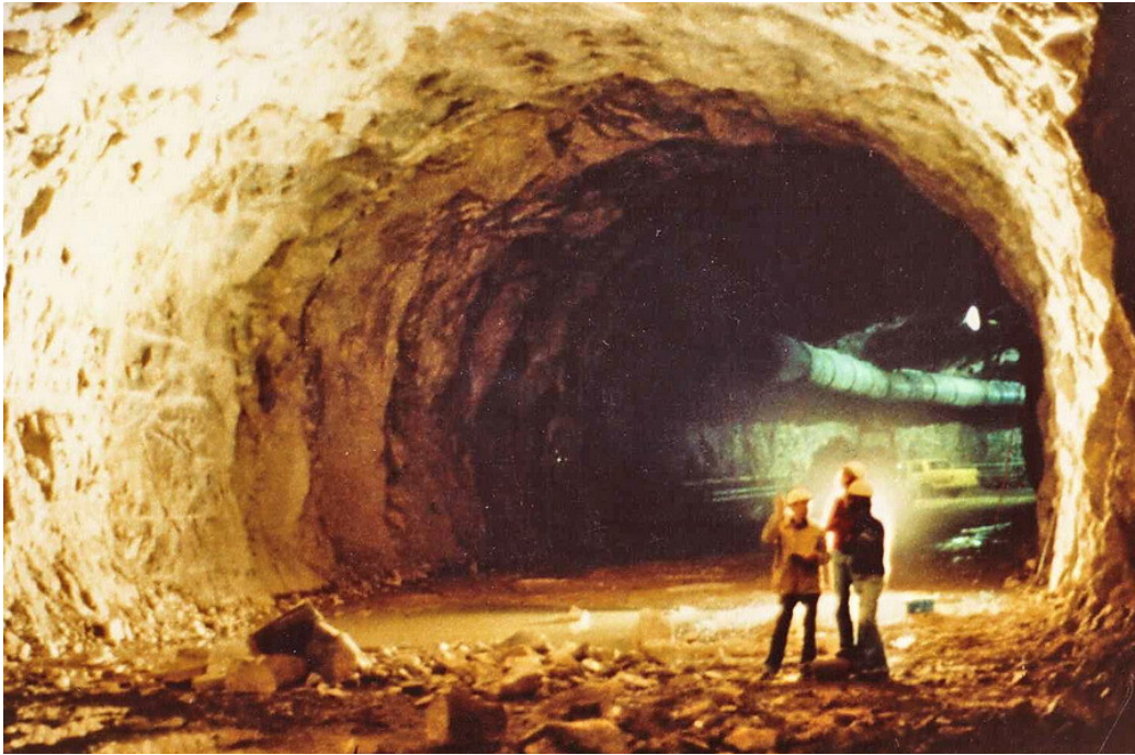
Figure 1: The 12 m span 8 m high top heading for the tailrace tunnel was constructed by full-face drill-and-blast and, because of the excellent quality of the massive gneiss, was largely unsupported.
